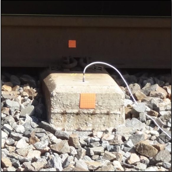
FIGURE 3 Miniature accelerometer attached to concrete tie.
