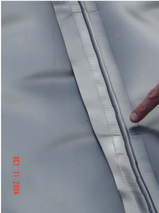
Figure 1. Air channel test performed in 0.75 mm PVC geomembrane seam.
