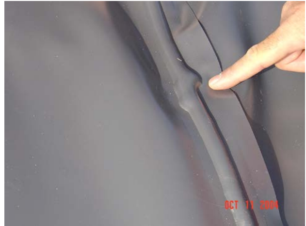
Figure 6. Aneurysm in 0.75 mm PVC geomembrane seam.
