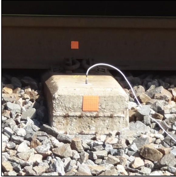
FIGURE 3 – MINATURE ACCELEROMETER INSTALLED ON CONCRETE TIE AT SITE 2
