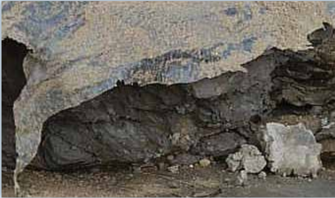
Figure 5. Close-up of torn geomembrane which shows slide surface is below geomembrane/CSL interface.
