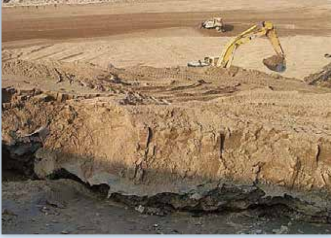
Figure 4. Slide surface and torn geomembrane.
