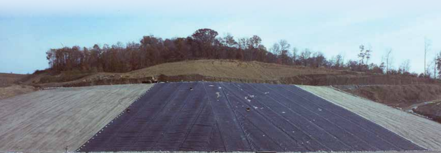
Figure 1. Slope overview and placement of geomembrane over completed low permeability compacted soil liner. (photo by Craig L. Walkenshaw)
