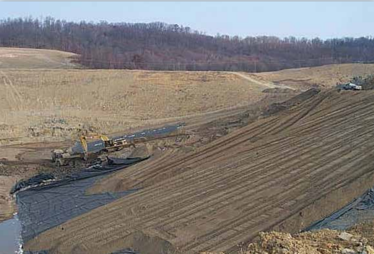
Figure 2. Overview of sideslope and protective sand placement on geomembrane from top of slope to bottom.
