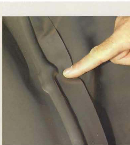
Photo 4. Aneurysm in 30 mil PVC geomembrane seam.
