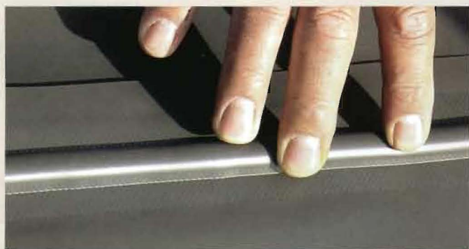
Photo 2. Inflated field seam in 0.75 mm (30 mil) PVC geomembrane.
