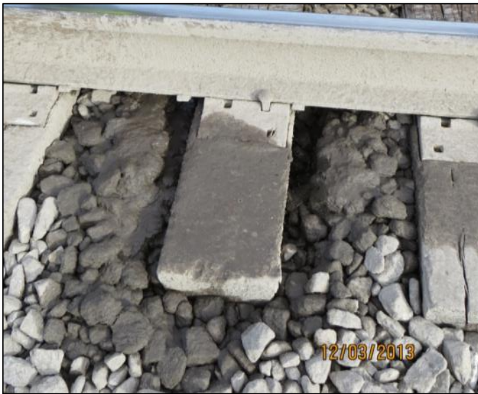
Figure 6: Photograph of wet, fouled ballast.
