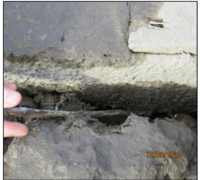
Figure 7: Photograph of a gap underneath a tie in a wet, fouled ballast section of track.
