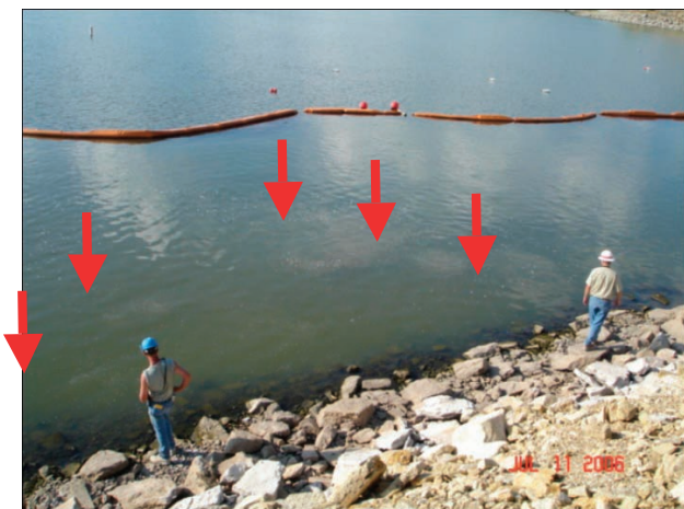
[FIG. 4] Photograph of air bubbling in Tuttle Creek Reservoir during jet grouting of upstream column S2-A3 with reservoir turbidity curtain in background
