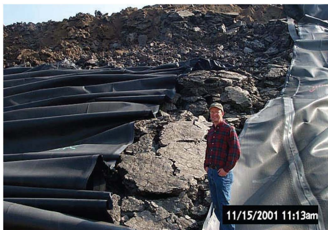
Fig. 3. Photo of failed slope and damaged geomembrane
