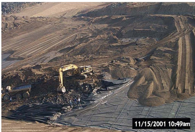
Fig. 1. Overview of failed slope and folded geomembrane at slope toe
