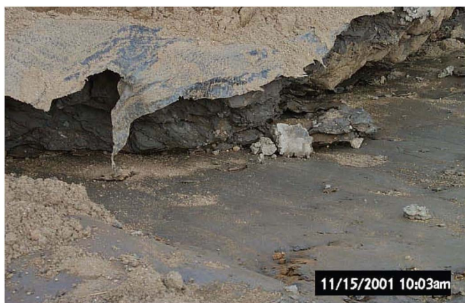
Fig. 5. Close-up of torn geomembrane that shows the slide surface is below the geomembrane/LPSL interface
