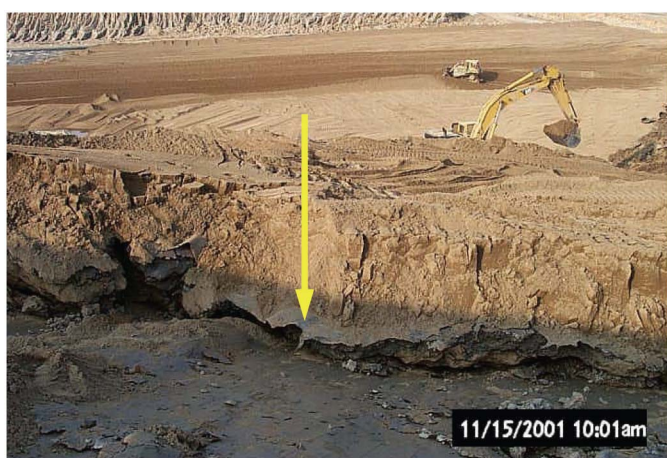
Fig. 4. Photo of slide surface and torn geomembrane
