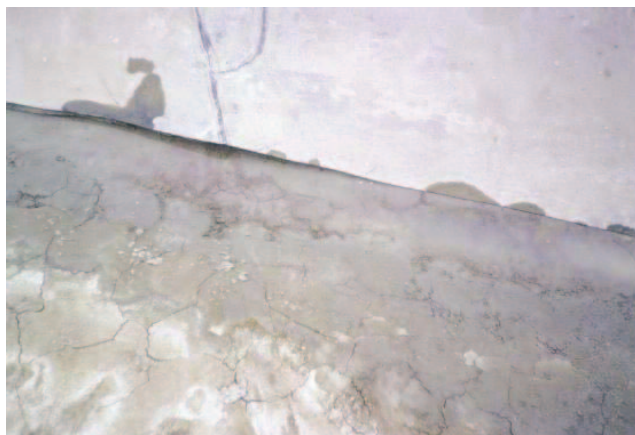
Figure 6. Close-up of hydrated bentonite accumulated on top of geomembrane on cell base after removal of overlying sacrificial geomembrane
