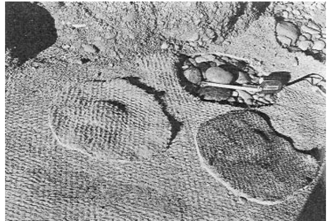
Figure 2. GCL overlying an incompatible subgrade (from Peggs and Olsta 1998)
