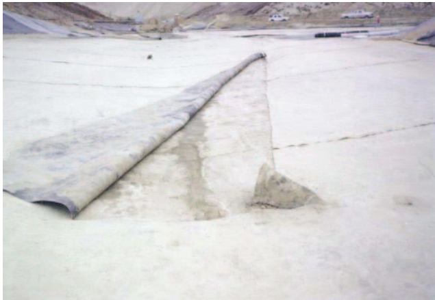
Figure 5. Layer of hydrated bentonite on top of geomembrane on cell base after removal of overlying sacrificial geomembrane
