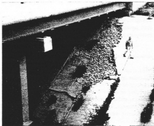
FIGURE 5 Damage to slope facing causing significant erosion of embankment soil.
