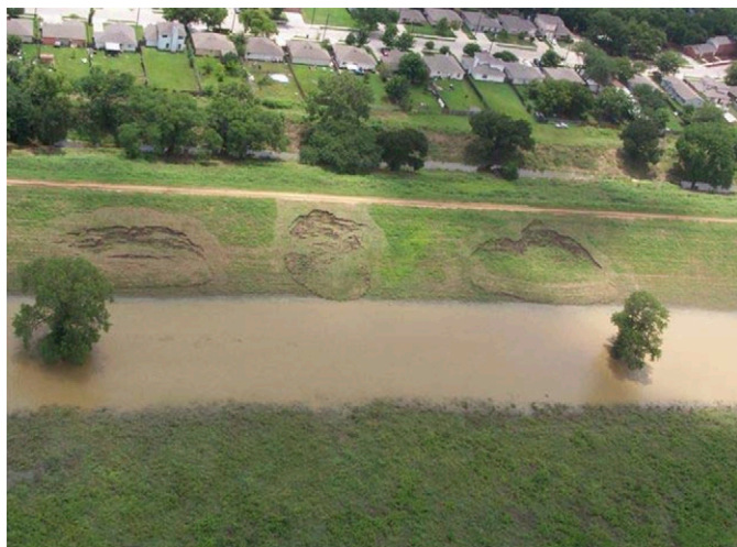
Fig. 1. Typical shallow slides in Dallas Floodway levee system with depths less than 2.5 m and widths from 27.5 to 36.5 m (photograph used with permission from USACE)
