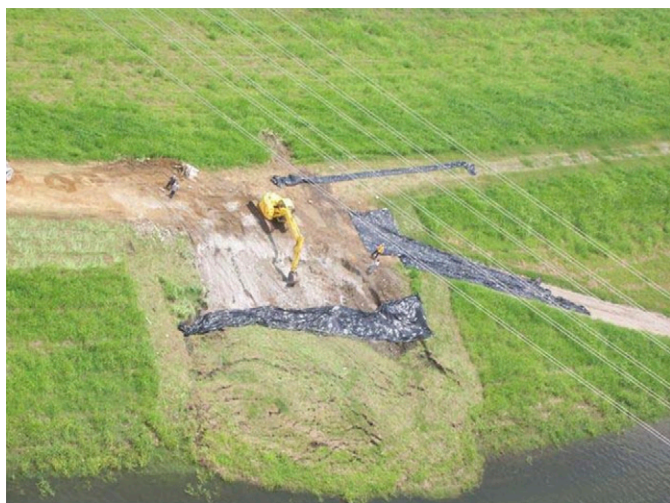
Fig. 2. Close-up of typical shallow slide in Dallas levees (photograph used with permission from USACE)
