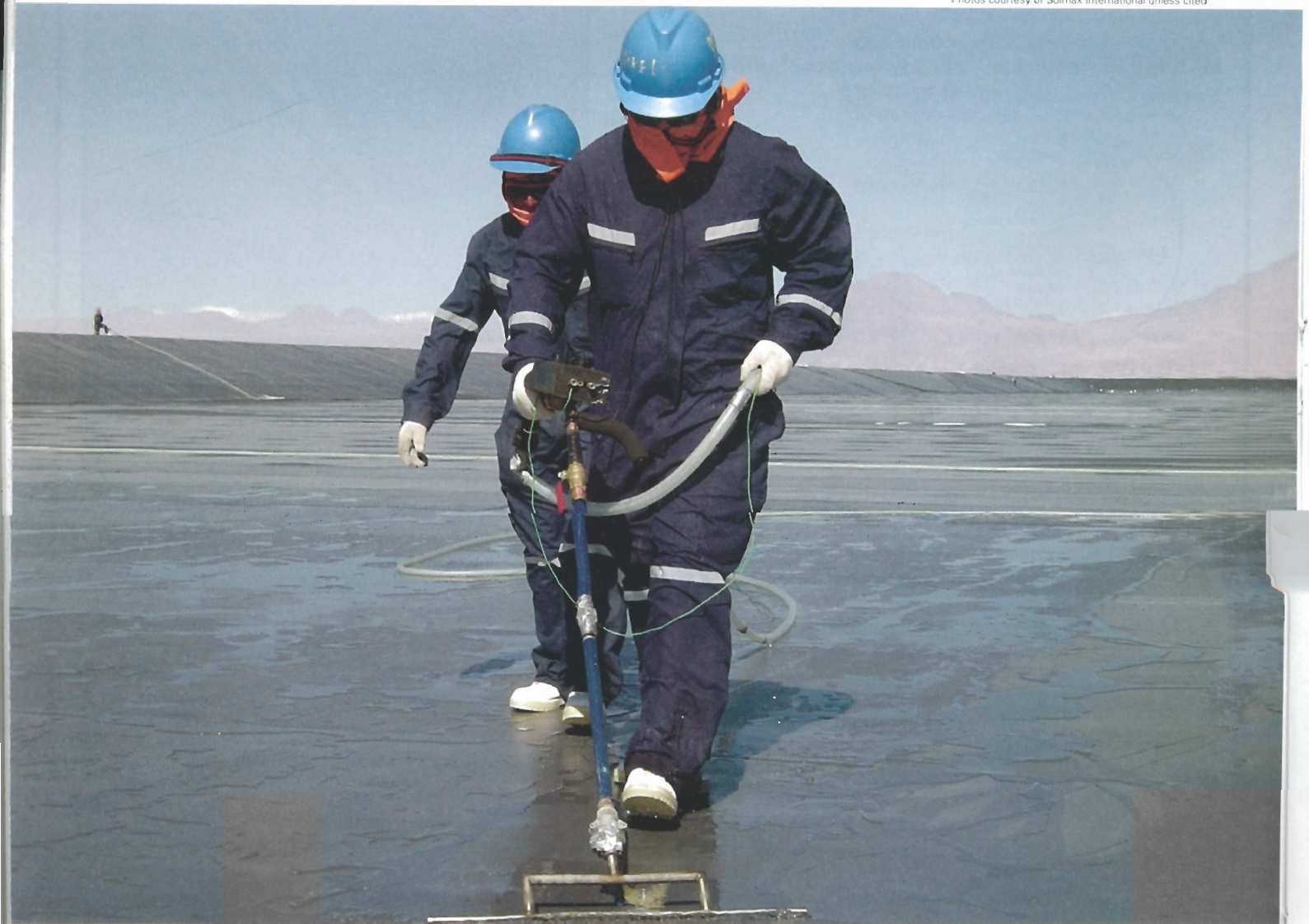
Photo 1 | In constructing the evaporation ponds, after the PVC liner is deployed, electrical leak-detection tests are done (see page 32).
