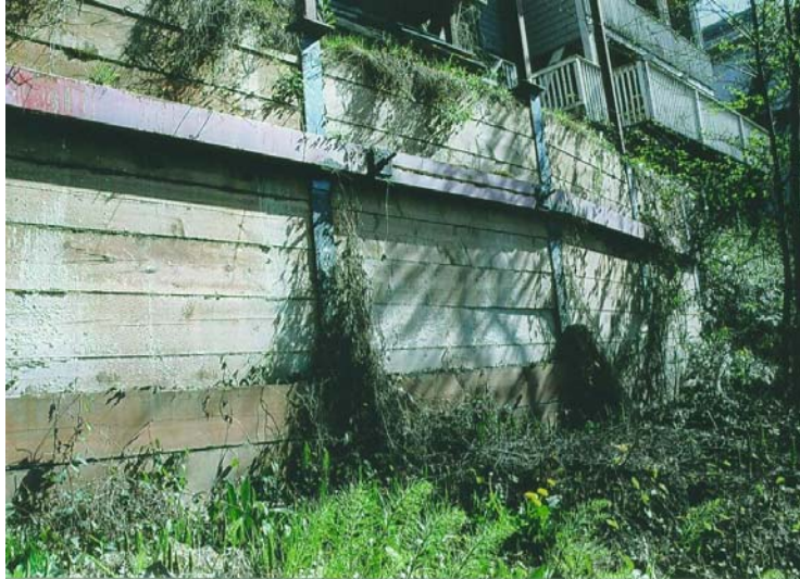
Figure 6: Existing anchored retaining wall system after nearly six years.
