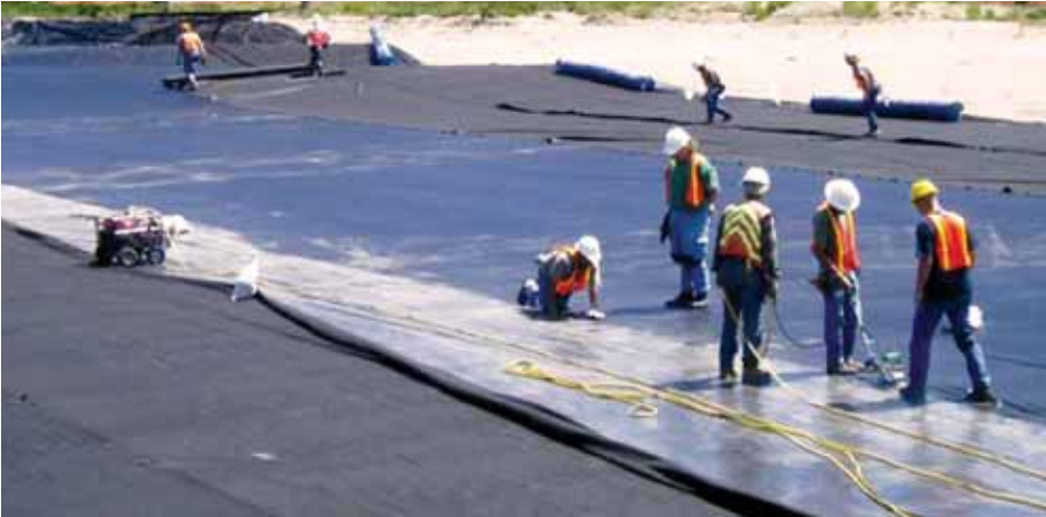
Photo 8 | Geotextile was deployed over a PVC panel while the panel is welded.
