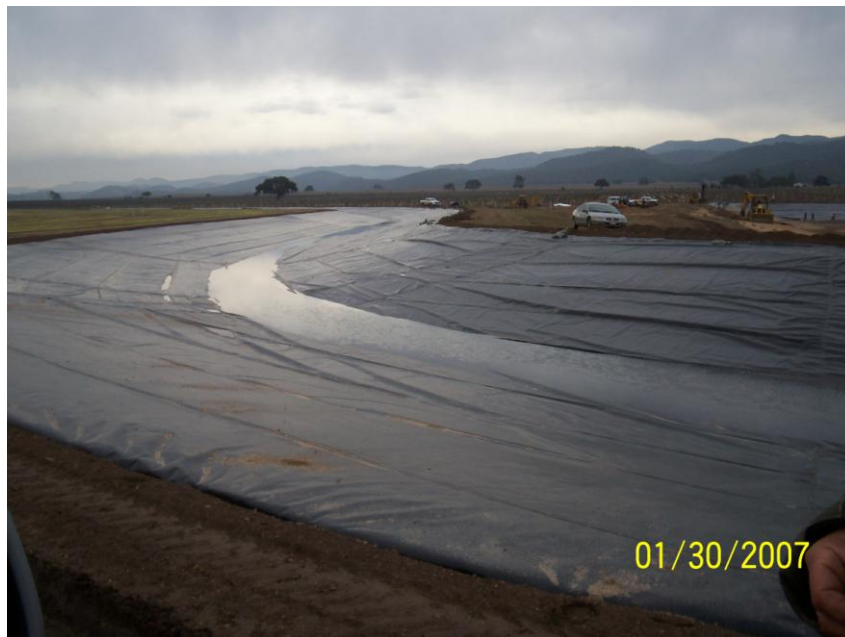
Figure 5 – Canal lined with a factory fabricated geomembrane
