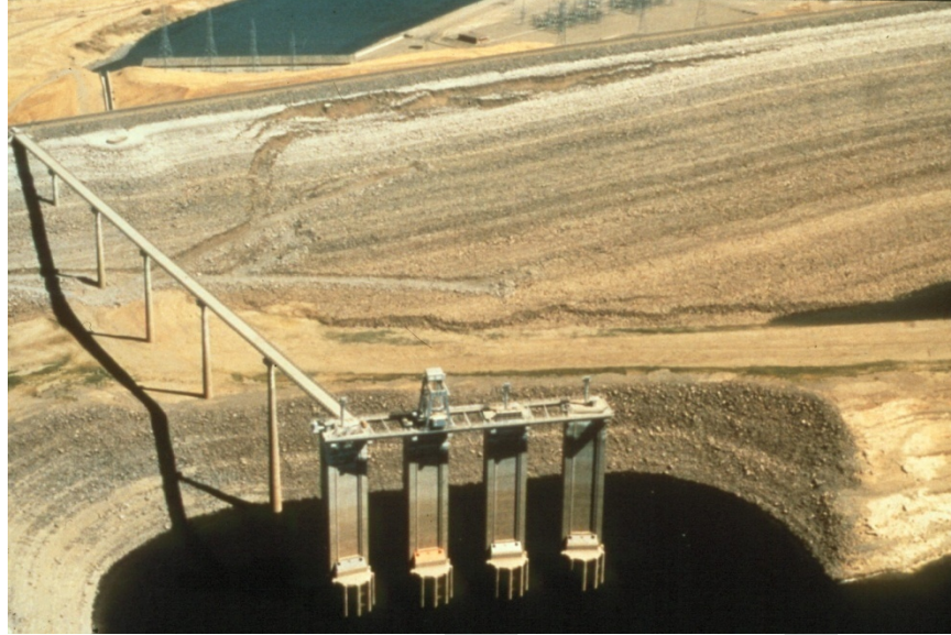
364 365 Figure 5. Slide in upstream slope of San Luis Dam in September, 1981 (photo from 366 California Department of Water Resources). 367
