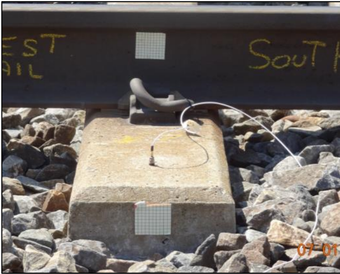
Figure 2: Photograph of a miniature accelerometer installed on a concrete tie
