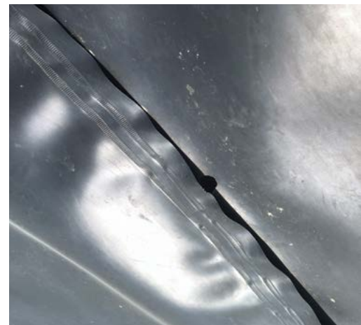
FIGURE 1 Close-up of damage to PVC geomembrane from deer hooves
